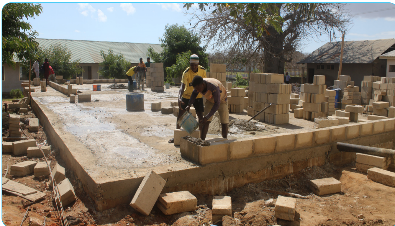
Fundis construct a classroom at Maweni Secondary School in Tanga Municipality, Tanga Region
